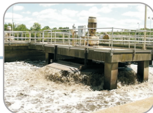
Effluent Treatment Plant
